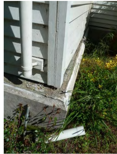
t) Foundation damage
