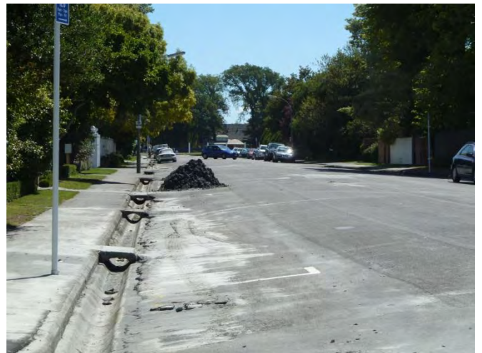
l) Liquefaction ejecta pile on road
