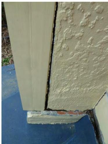
u) Foundation damage
