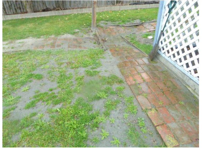
h) Undulations in lawn, liquefaction ejecta removed
