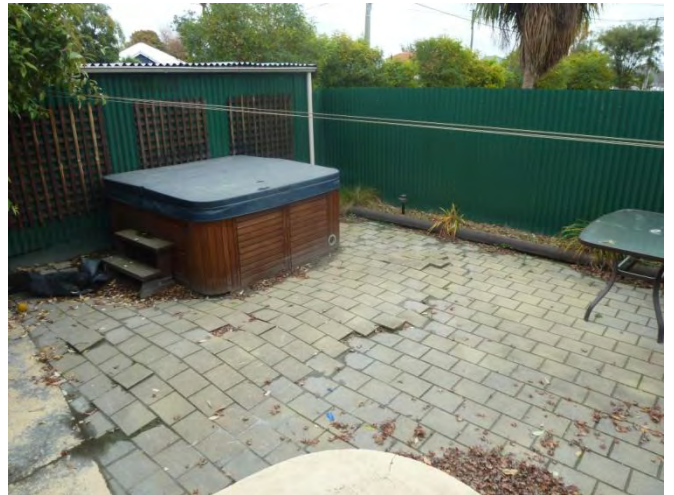
d) Undulations in paving area
