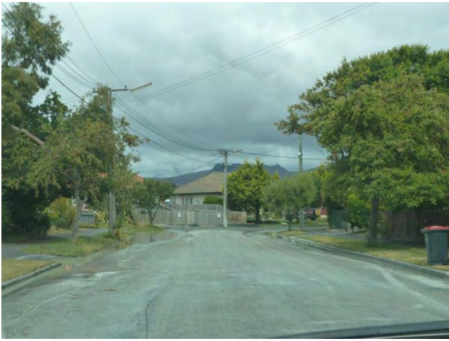
y) Undulations on road with ponding water
