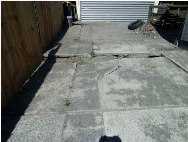
s) Undulating paving slabs
