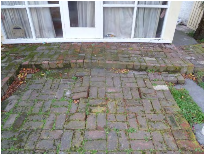
a) Undulating paving bricks
