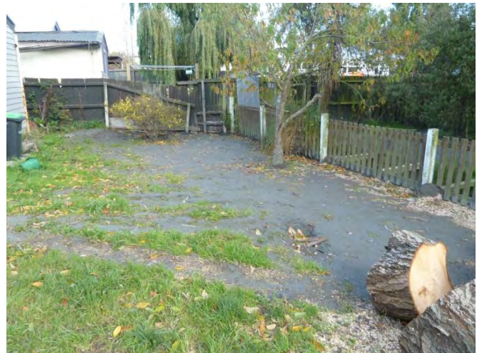
d) Liquefaction ejecta on lawn
