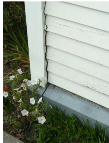
f) Foundation damage
