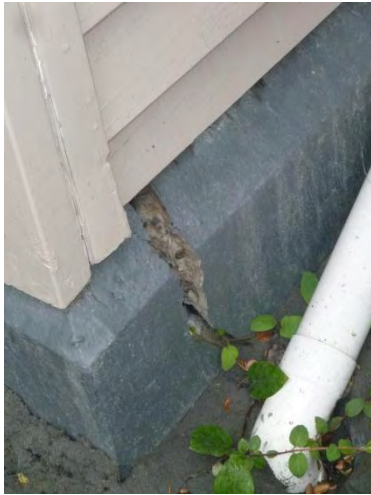
o) Foundation damage
