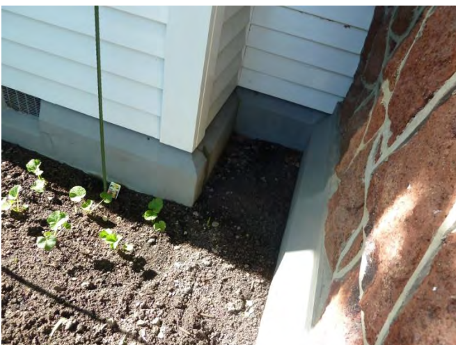
w) Foundation damage
