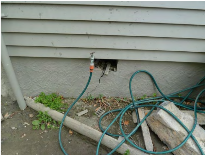
i) Foundation damage
