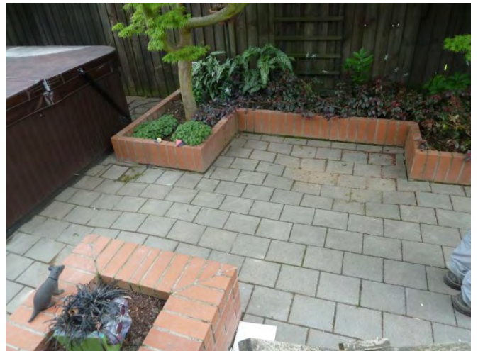
v) Undulating paving slabs
