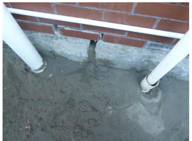
f) Foundation damage
