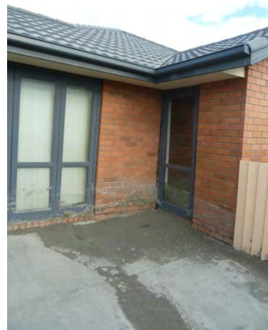
p) Outside of dwelling showing level liquefaction ejecta reached on brickwork and windows
