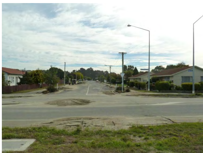
w) Liquefaction ejecta at a New Brighton Road junction
