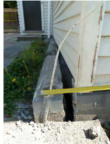
v) Foundation damage
