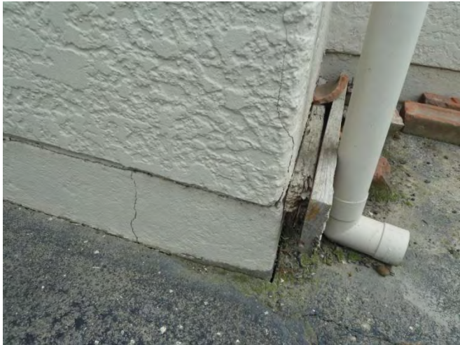
c) Foundation damage
