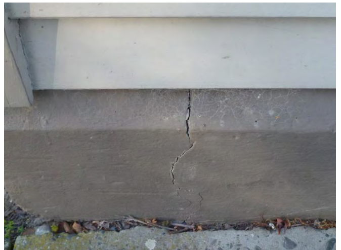
f) Foundation damage
