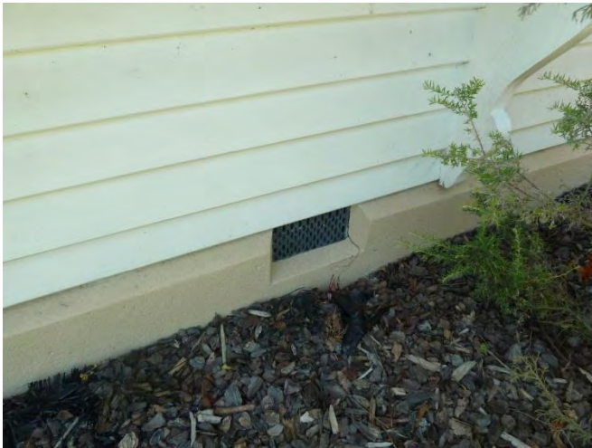
c) Foundation damage
