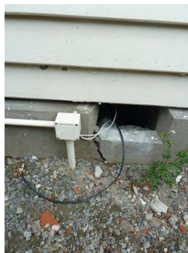
t) Foundation damage
