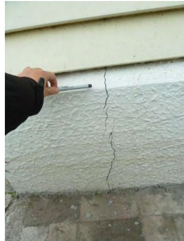
d) Foundation damage
