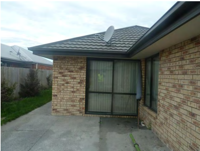
o) Foundation damage, dwelling tilting
