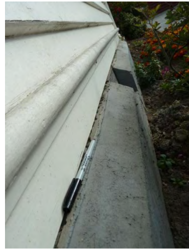
n) Foundation damage
