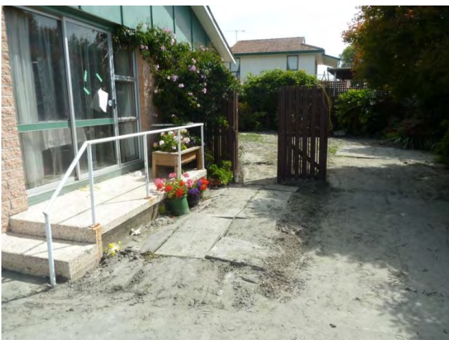
e) Undulating paving slabs with liquefaction ejecta
