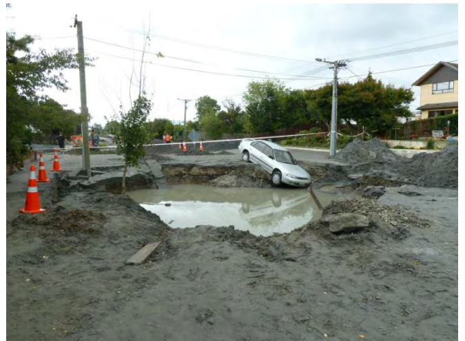
r) Close up photo of road damage seen in aerial photo of Woolston
