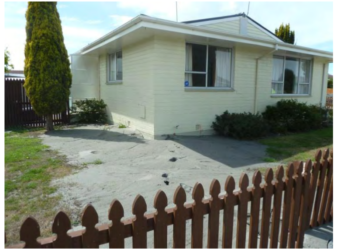
b) Large patch of liquefaction ejecta
