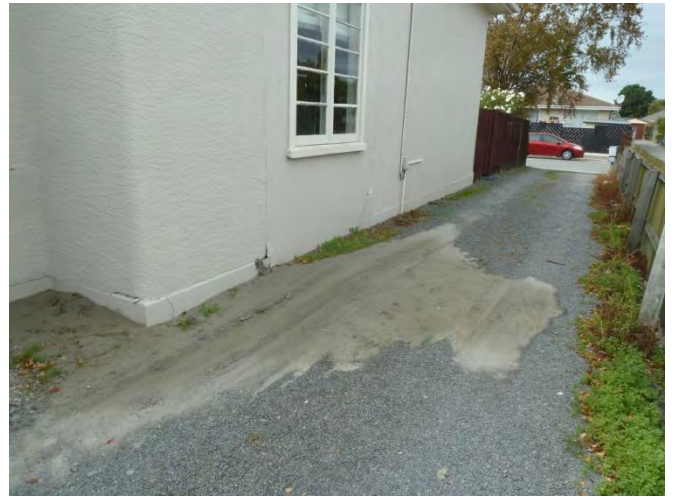
b) Isolated area of liquefaction ejecta
