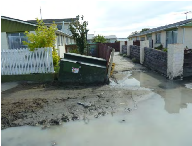
y) Sinking electricity box with liquefaction ejecta and ponding water
