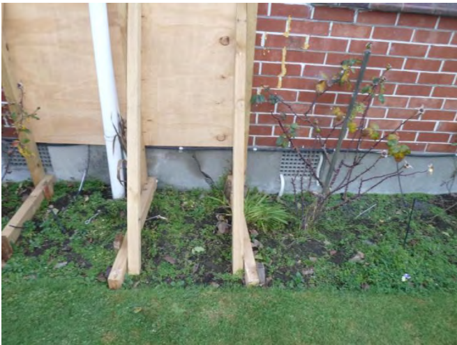
u) Foundation damage
