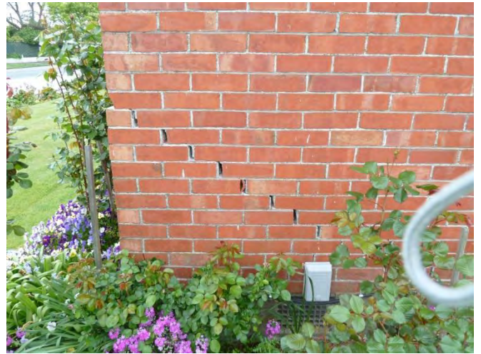
t) Damage to brickwork
