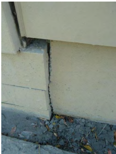
e) Foundation damage
