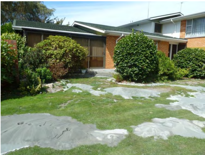
c) Numerous patches of liquefaction ejecta
